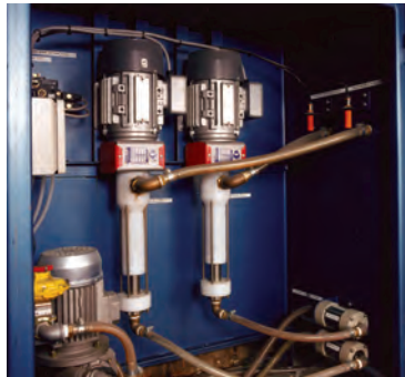
2 LF pumps delivering sulphuric and sulphonic acid at a steady and consistent flow
